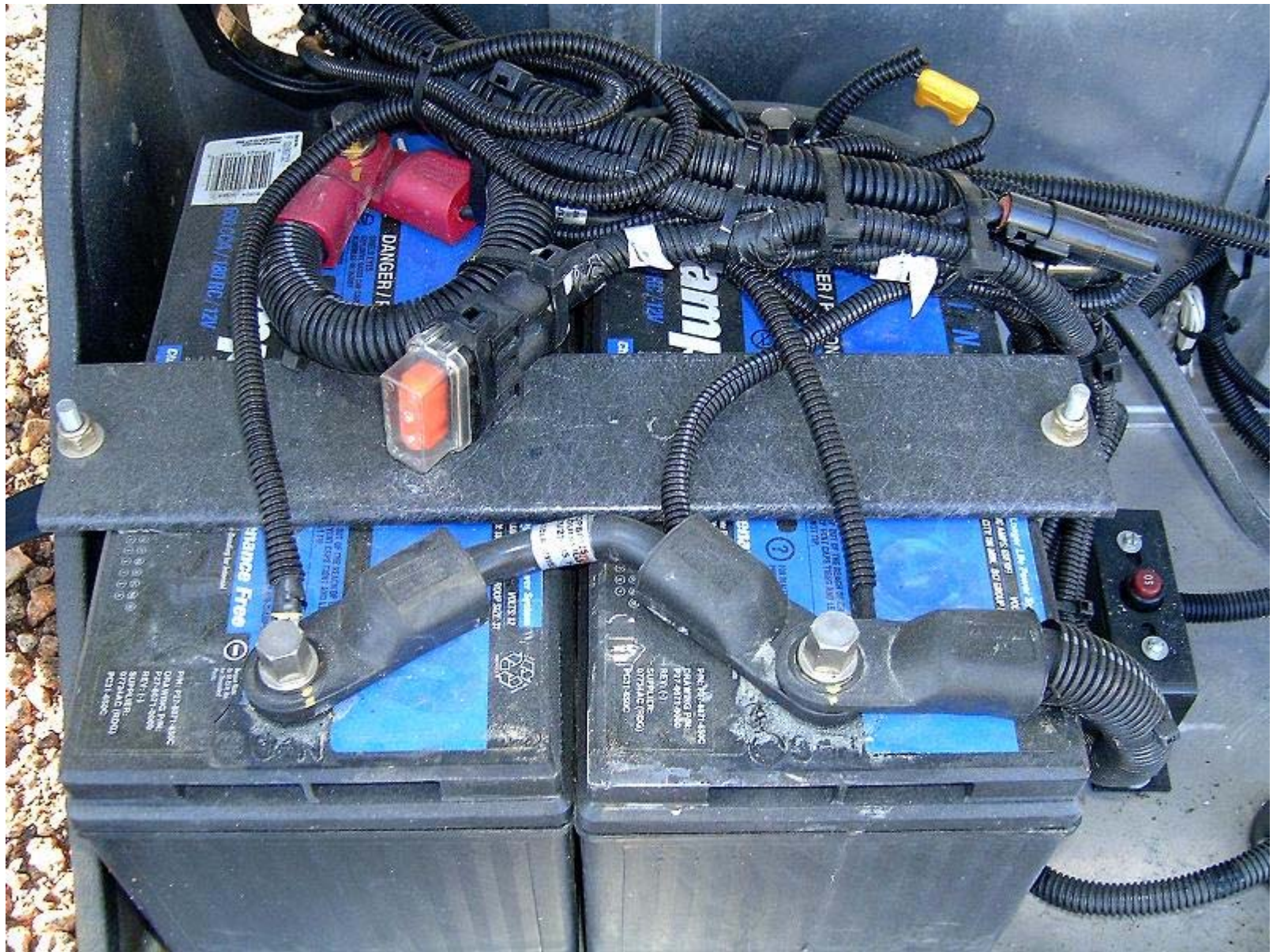
Junction Box Connection to Battery
