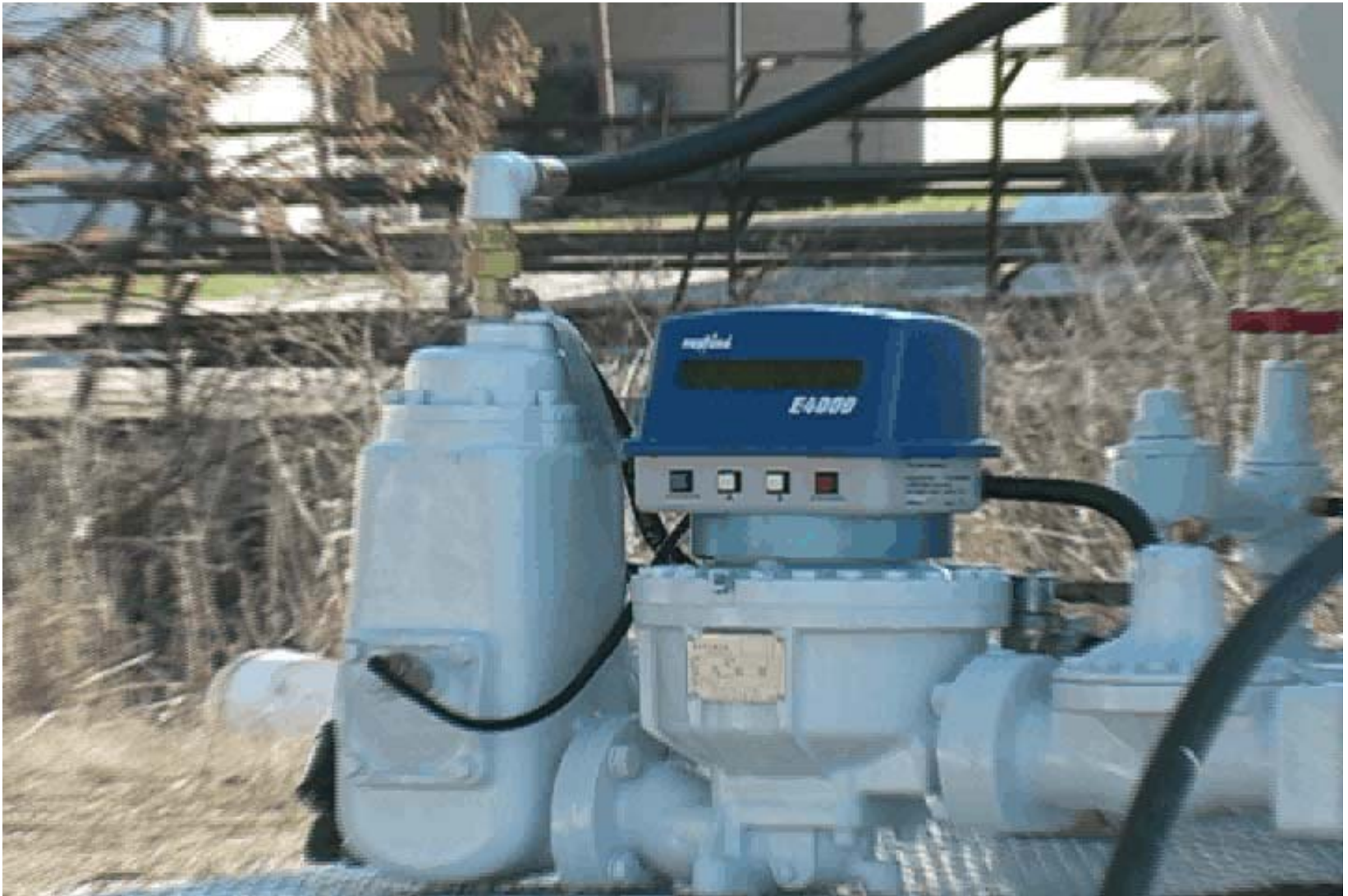
Installed on Mechanical Meter
